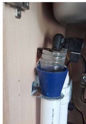
Figure 2 - Tundish with air gap obstructed
