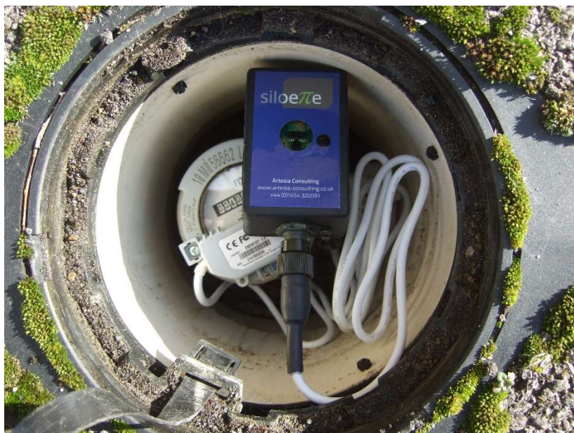
Figure 3 Siloette logger installed in a boundary box
